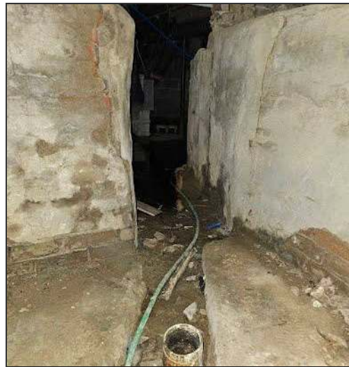
Open clean-out + hose in trench Cap removed (report language).
