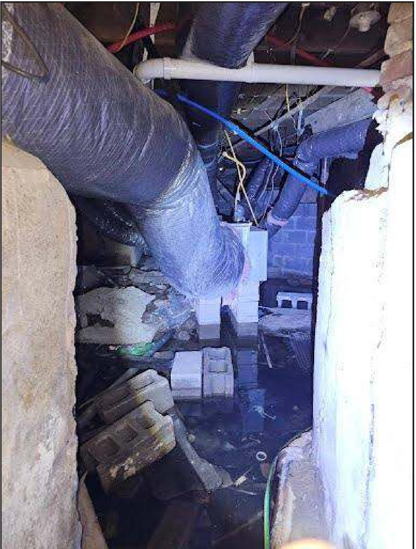
Furnace bay — heat plant on stacked CMU above flood water
